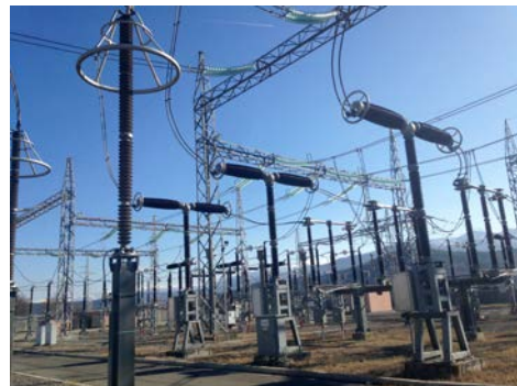
Modern substation in Elbasan, Albania.
